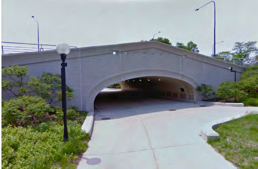
Existing Pedestrian Underpass at Hayes Drive/63 rd Street beneath Lake Shore Drive
